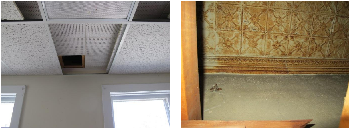
Figure 02. Two layers of dropped ceilings conceal the original tin ceilings in at least two rooms at the second floor.
