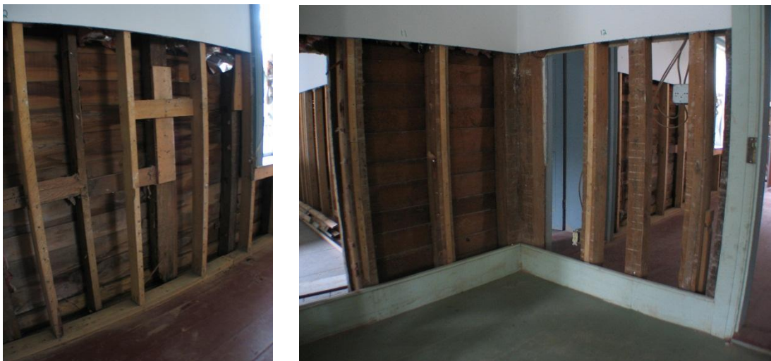
Figure 06. Images show typical variations on stud wall framing. Image on the left shows an exterior wall with a newer interior stud wall added to provide a new cavity for insulation and to re-plumb the interior wall surface; image on the right shows typical original stud framing, with original door and base trim left in place and used as a guide for edges of the new gypsum board walls.
