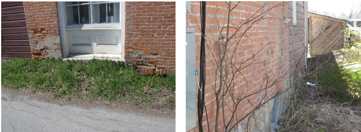
Figure 12. Image on the left shows area of brick spalling and attempted repair using hard portland cement mortar. Cement-based mortars are generally incompatible with historic lime-based mortars and tend to cause more accelerated deterioration of the masonry assemblies they are meant to repair. The image on the right shows significant settlement and bowing of the masonry wall within the last 6'-0" +/- as it approaches the intersection with the timber-framed addition.
