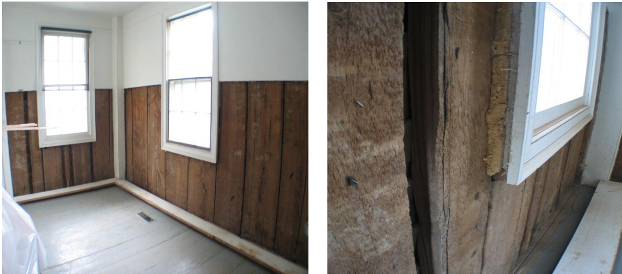
Figure 05. Image on the left shows an example of the unique plank wall sheathing at the former bank building, which was moved and attached to the Pratt Museum. Image on the right shows remnants of foil-faced 1" polyisocyanurate board insulation below ½" gypsum board fitting behind the trim surrounding the window opening.
