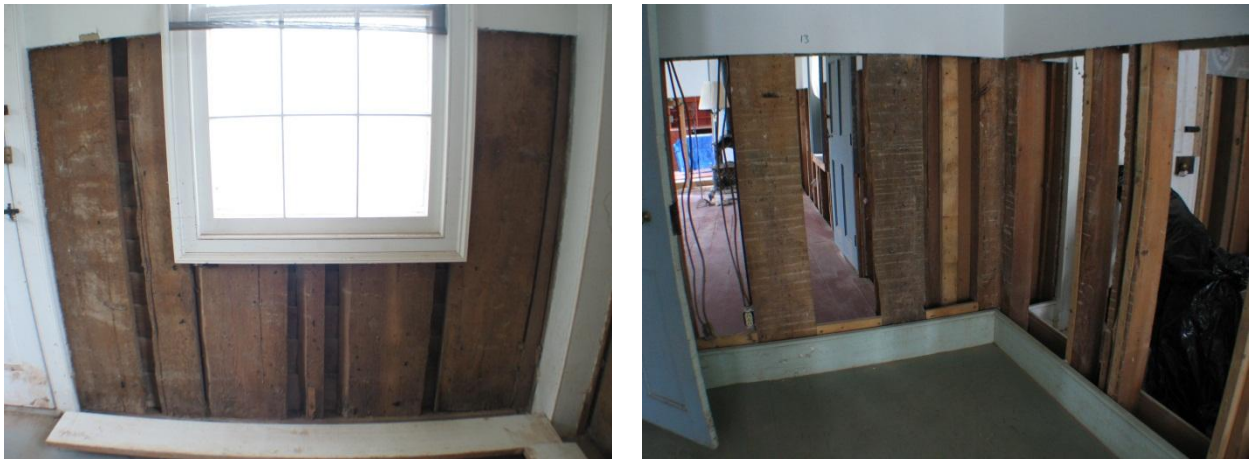
Figure 16. Image on the left shows an exposed section of the exterior plank wall construction in the bank window. Image on the right shows the intersection of a more common interior stud wall framing condition in the original footprint with a modified version of the plank framing used in the bank wing.
