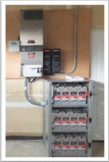
28. Battery Back-Up Photos - Photo showing battery back-up system and racking.
