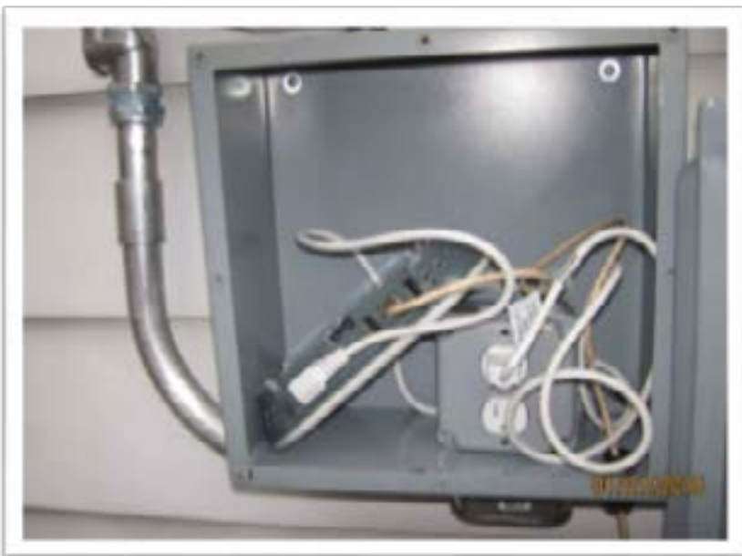
Photo D9: Equipment is not rated for location. In this case, a non-GFCI outlet for PV monitoring equipment is located in a wet location: NEC 110.3(B), 210.8(A)(3)
