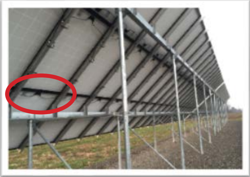
Photo D5 - Conductors over 30V not guarded, installed in raceway, or otherwise inaccessible: NEC 690.31(A)
