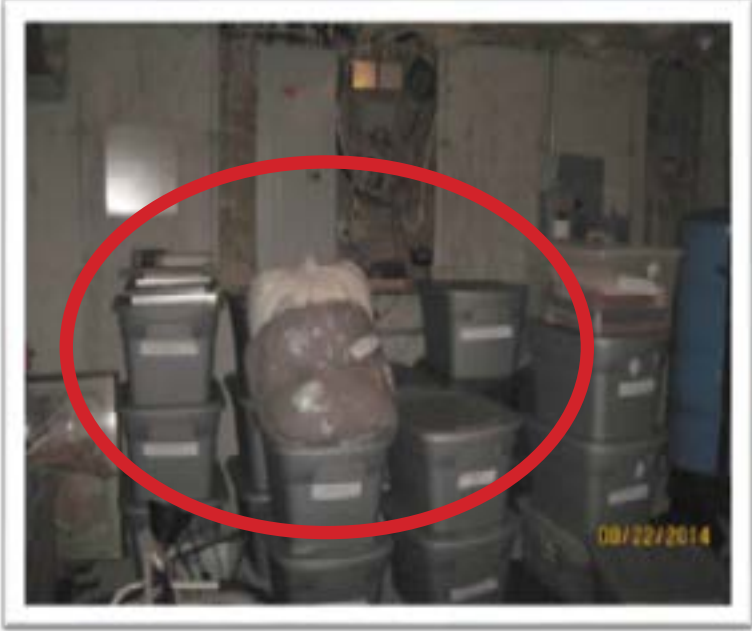
Photo D3: Working clearance not maintained: NEC 110.26
