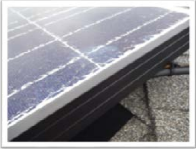
Photo D4: Equipment visibly damaged
